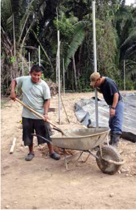
One of the breeding ponds just after liner installation and before being filled with water. Note the uprights of the perimeter fencing under construction in the back. PHOTO CREDIT: JACOB MARLIN
